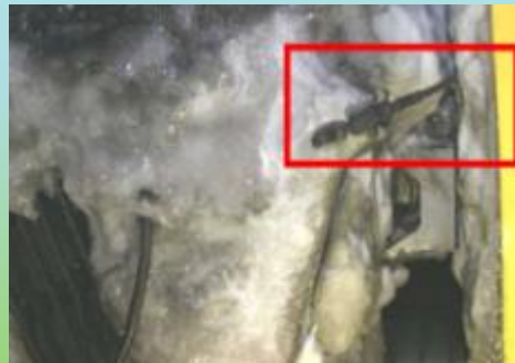
Protection of the cabling
