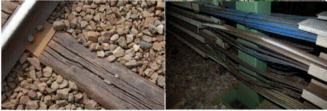
Figure 1 Railway infrastructure is constituted of large amounts of material, such as rails, sleepers, ballast, cables and different construction elements.
